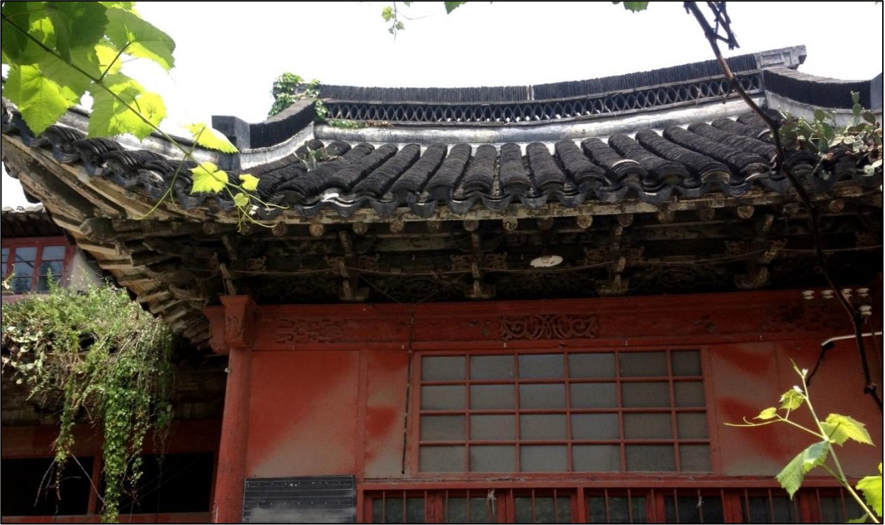
Fig. 13 – Lao Tang in 2013 (Photo by S. Piastra). Currently, the former church, deconsecrated after the rise of the People's Republic of China, is annexed, in critical structural conditions, to a primary school of Shanghai's 'Old City'. A restoration and regeneration of it into a museum, focused on China's cultural encounter with the West, are warmly recommended. On the lintel, above the window, a stylized 'M' stands for Holy Mary, to Whom the church was dedicated in the last decades of its consecration.
