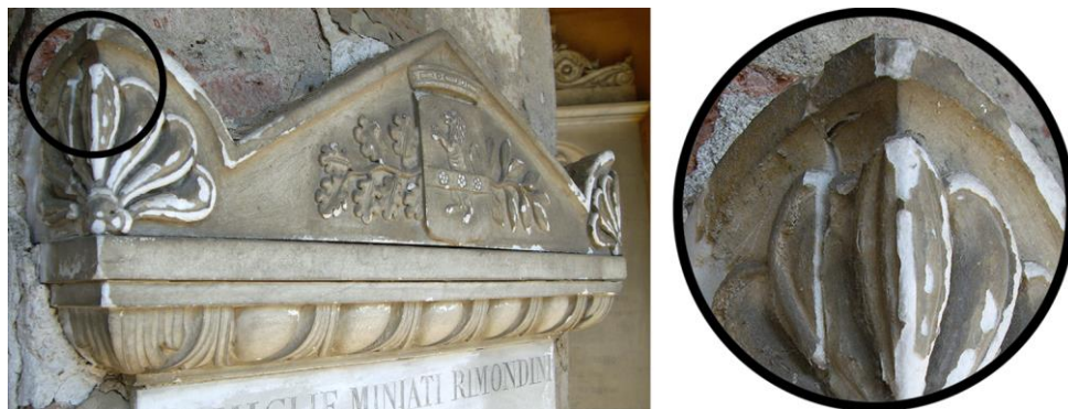
Figure 1: Example of marble decoration affected by sulfation (Monumental Cemetery in Bologna, Italy, XIX century). Beneath the gypsum surface layer (also incorporating some particulate matter), marble exhibits grain disaggregation
