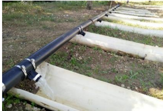
Figure 18: Egypt: Self-compensating gated pipe system
