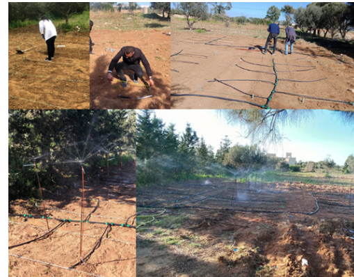
Pilot plant P2 for textile wastewater treatment and reuse in Nabeul, Tunisia: installation of the irrigation system in the experimental field
